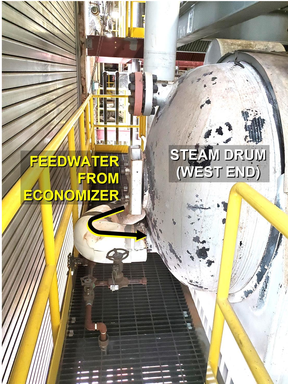
Figure 21 – Feedwater Supply to Steam Drum (West End)
